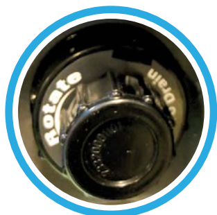
External drain valve
